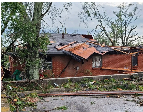
A family's home, its roof torn open and the yard full of downed trees. Courtesy Lori Elizabeth Grayban.
