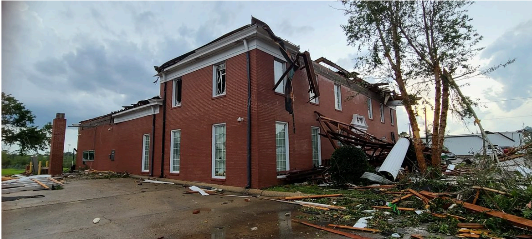
Merchants & Marine Bank on Main Street, its roof torn away. Courtesy Lori Elizabeth Grayban.
