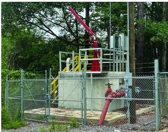
A rebuilt sewer pump station, raised above the flood line so rising water can no longer drown it. Courtesy Neel-Schaffer.
