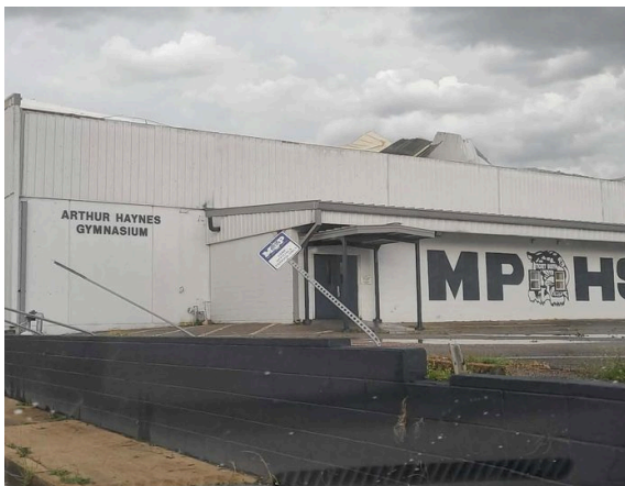
The Arthur Haynes Gymnasium at Moss Point High, its roof lifted while students sheltered inside. Courtesy Lori Elizabeth Grayban.
